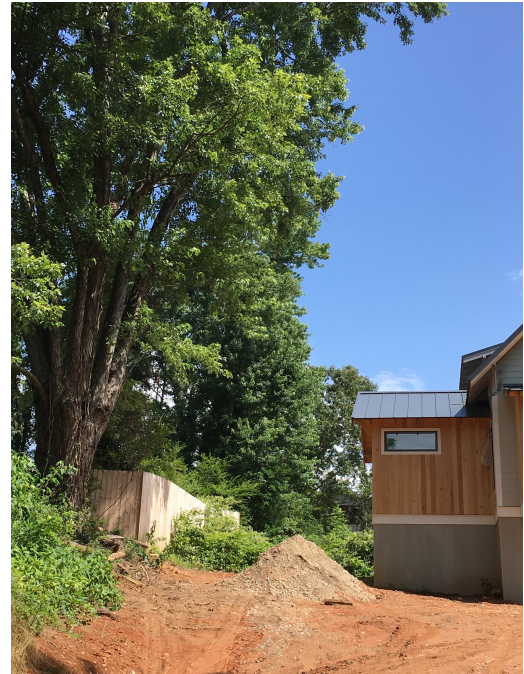
Trees on or near property lines (boundary trees) are often damaged from the construction activities on the adjacent properties.
